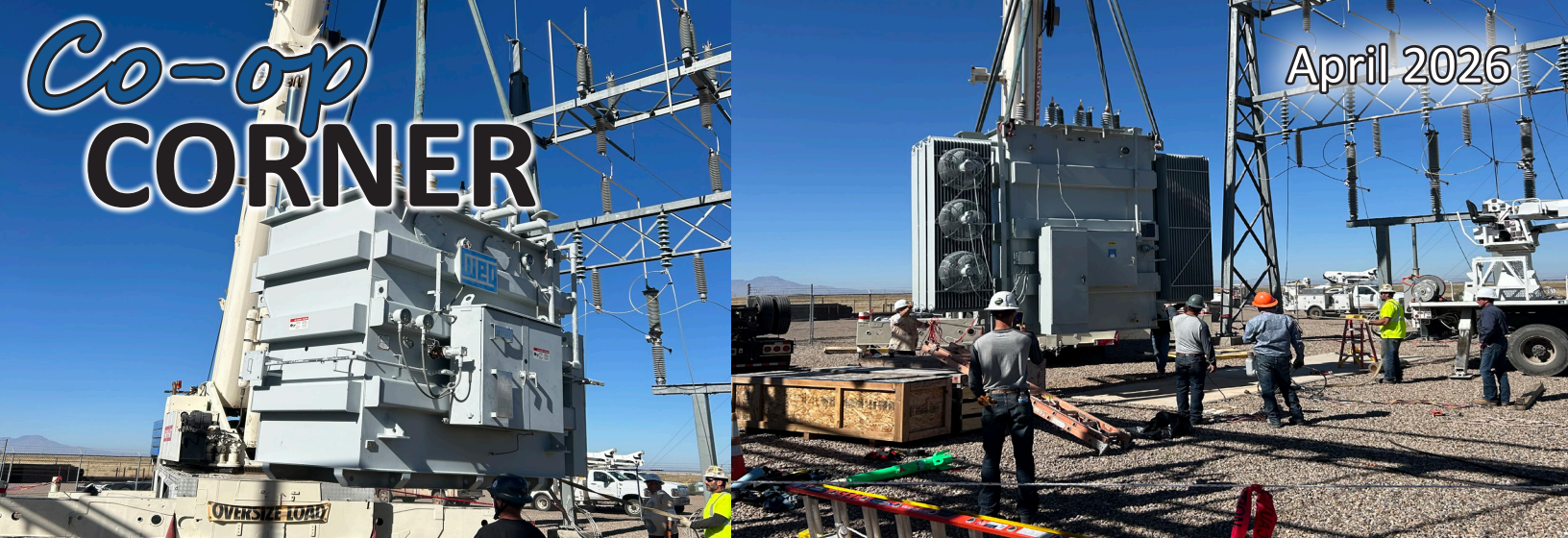
"Out with the old, in with the new" - SEC Line Crews replacing the Burris Substation transformer
