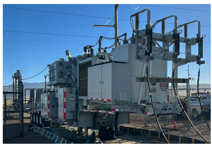
Our partner Tri-State G&T provided their Mobile Substation which was invaluable to the success of this project!
