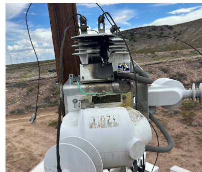
Damaged Pole Top Metering CT
