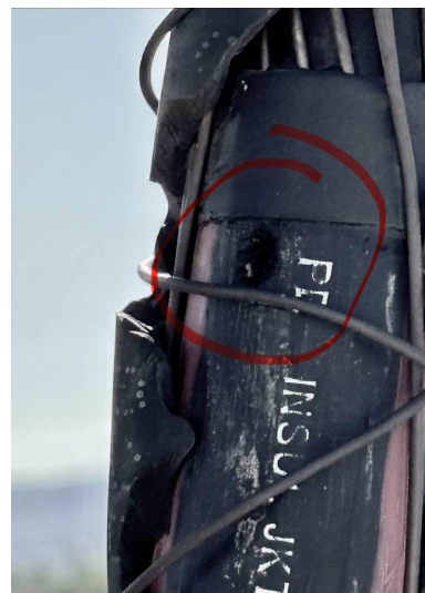
Pinhole damage to UG takeoff
